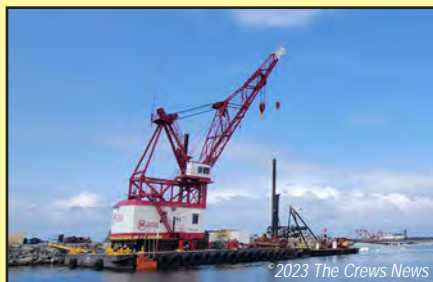
April 2023 - Manson's crane ready to help. Dredge at work in the background.
